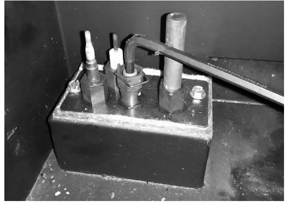
Figure 7 – Loosening Pilot Orifice
