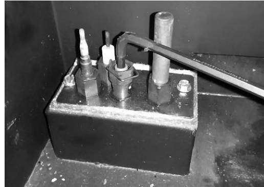
Figure 7 – Loosening Pilot Orifice
