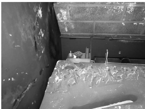
Figure 10 – Pilot, Shield, and Burner Position
