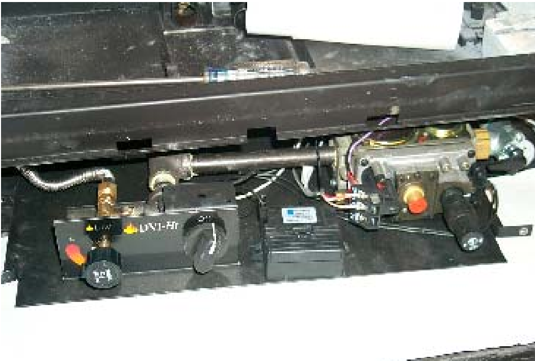
Photo 9 Valve tray pulled out for service.
