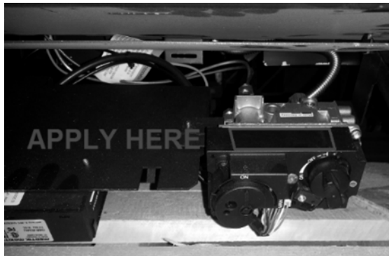
Figure 20 – Valve Warning Label Location
