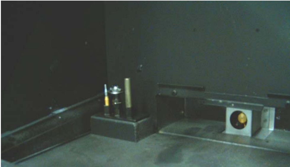
Photo shows Pilot assembly (left) and air shutter with burner orifice (right) in the firebox after the pan burner is removed.
