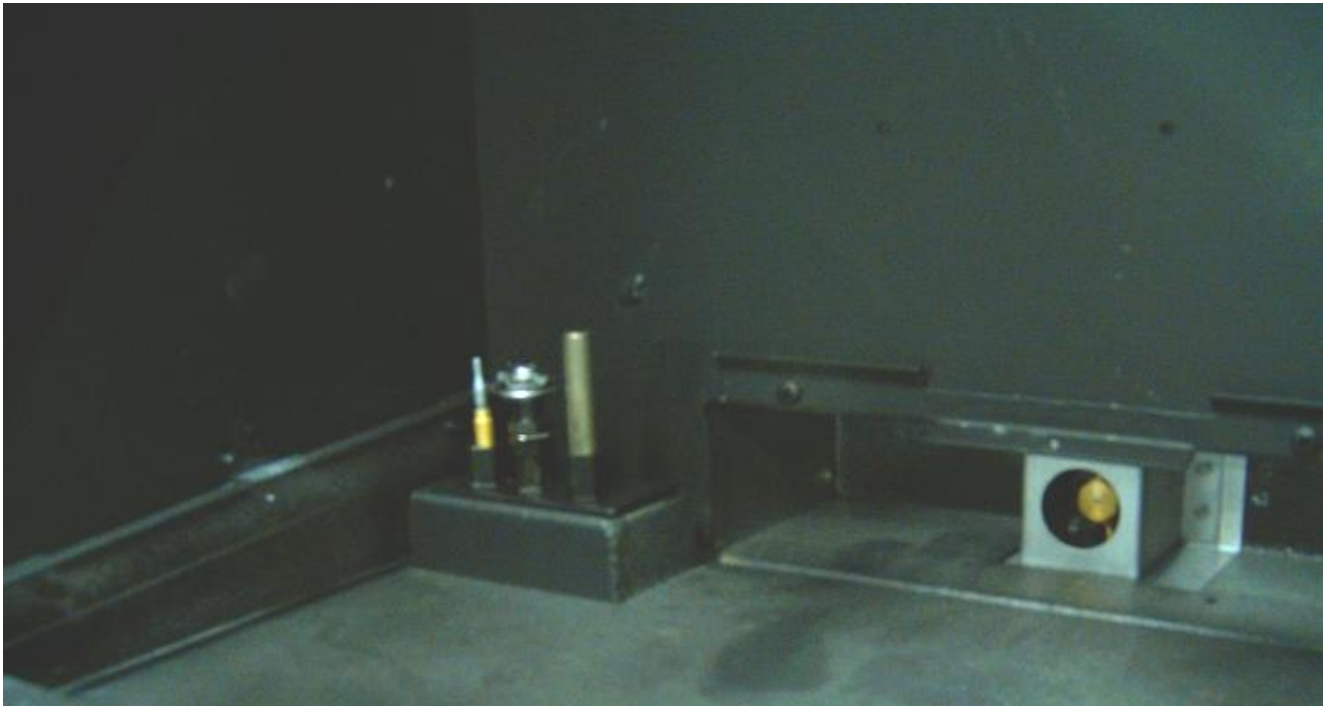
Photo #4 Pilot assembly (left) and air shutter with burner orifice (right) in the firebox after the pan burner is removed
