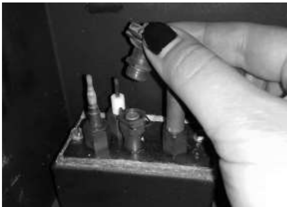
Figure 7 – Removing Pilot Burner Hood
