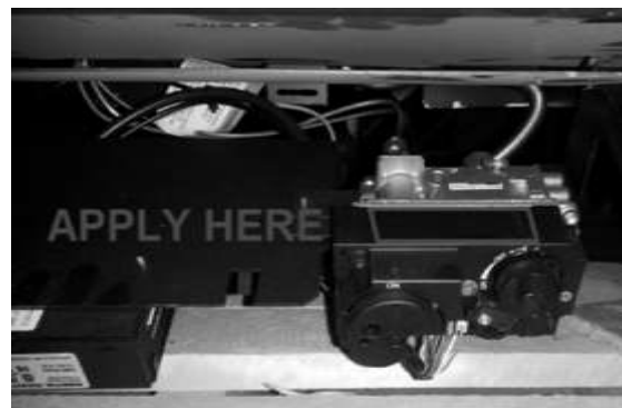
Figure 17 – Valve Warning Label Location
