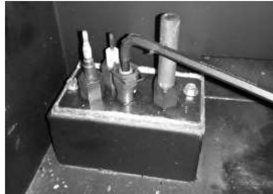
Figure 8 – Loosening Pilot Orifice
