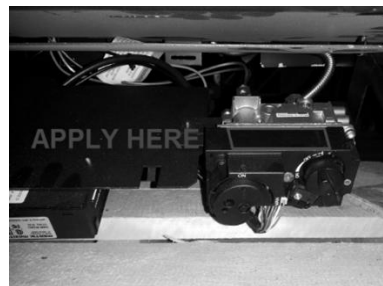
Figure 22 – Valve Warning Label Location
