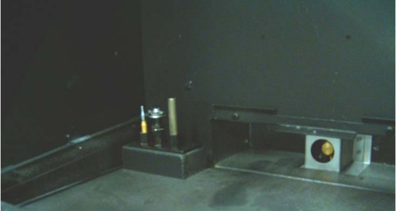
Photo shows Pilot assembly (left) and air shutter with burner orifice (right) in the firebox after the pan burner is removed.
